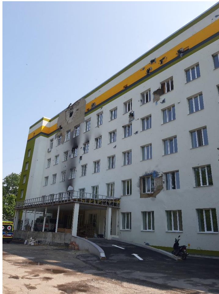
Pic. 3. Damage to exterior of the Trostyanets City Hospital. Captured by UHC with the eyeWitness to Atrocities app. Item ID 133743. See Annex I.
